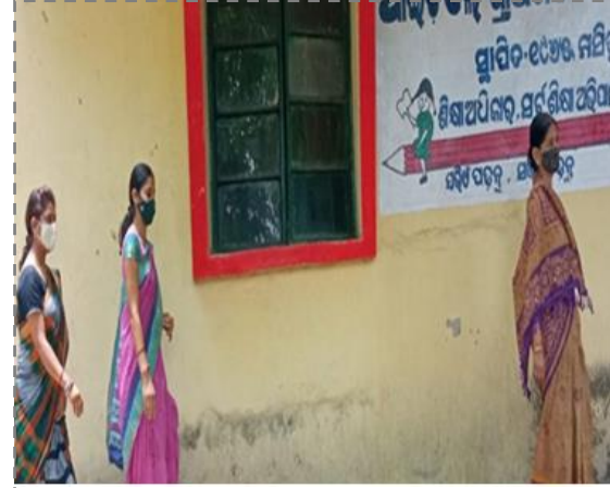
Modification & renovation of IDL Primary School has been going on. In this course the students from nearby villages are benefited
