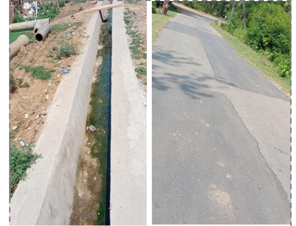
Repairing of IDL Road from & construction of adjacent drain. Villagers of Balijhudi & Sonaparbhat are benefited with this repairing work
