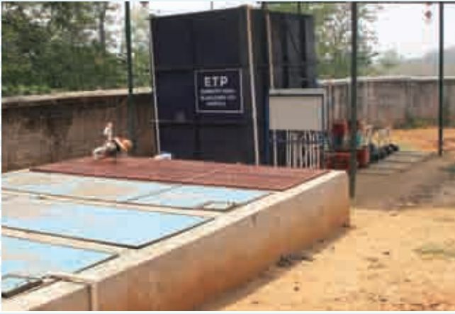
Effluent Treatment BIO-Plant at Rourkela
