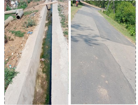
Repairing of IDL Road & construction of adjacent drain. Villagers of Balijhudi & Sonaparbhat are benefited with this repairing work
