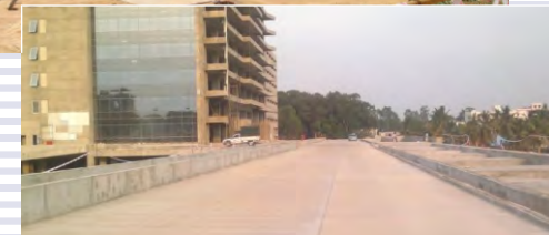
Elevated road work completed in the 40 acres Ecopolis (SEZ) at Yelahanka, Bengaluru
