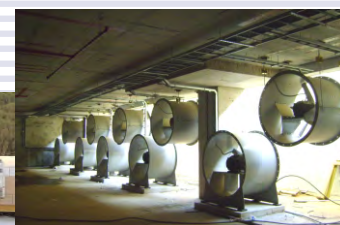
Cooling and ventilation systems
