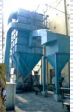
Pulse jet bag filter system installed at Hyderabad
